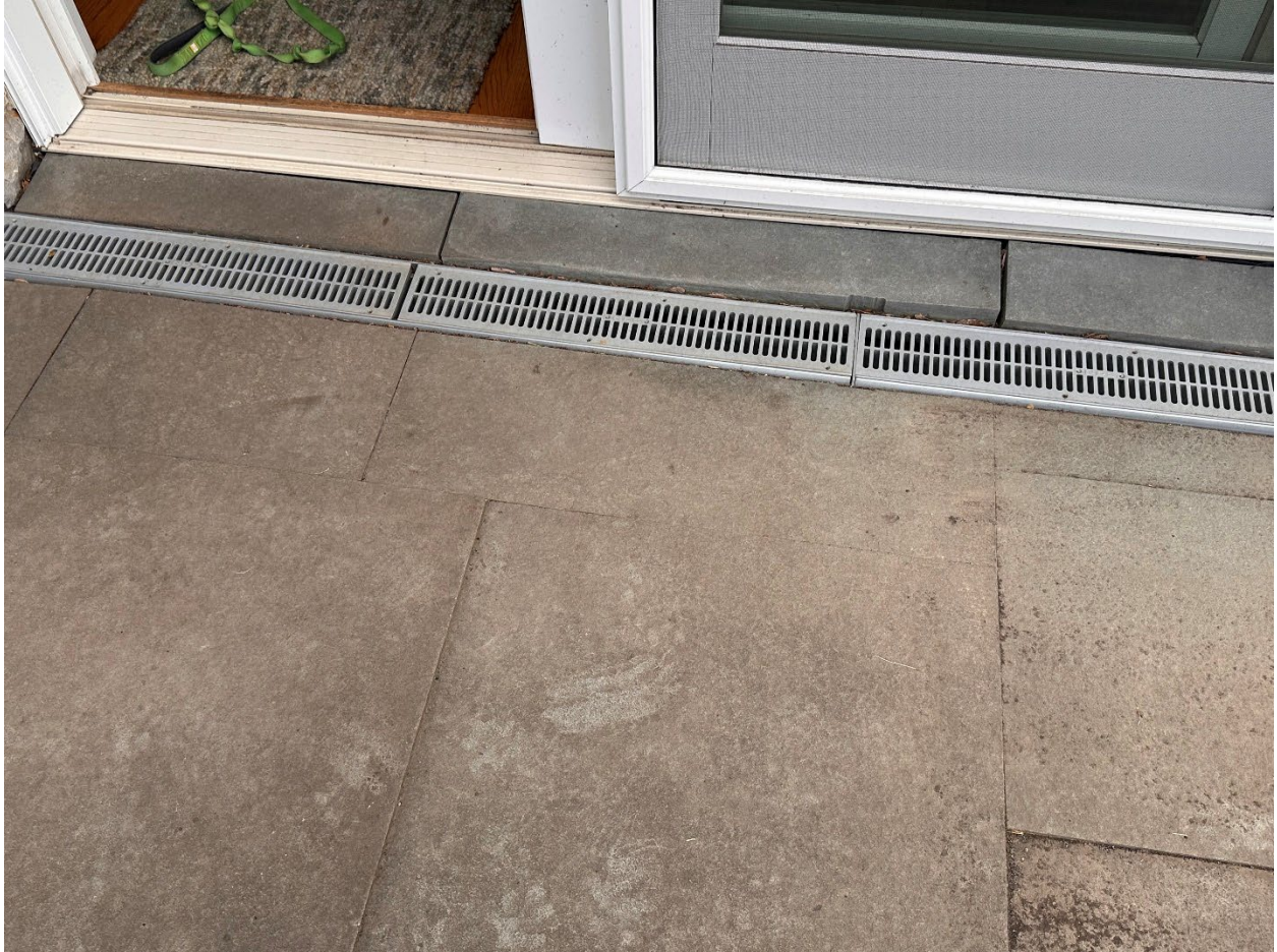
Photo 11; flush drainage system just outside the back door
